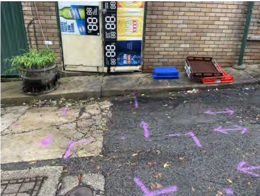
Photograph 6: Image of the approximate location of the UST and service locating showing potential underground piping, looking east (dated 5 June 2024).
